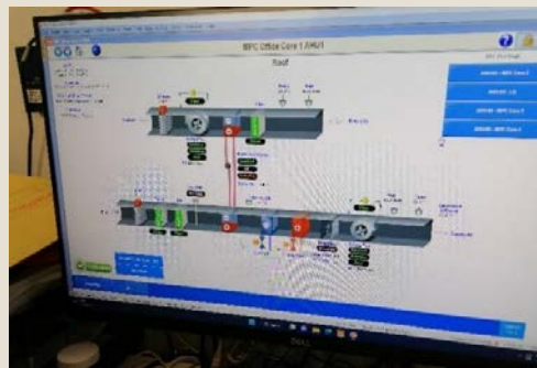
BMS screen display at Here East
