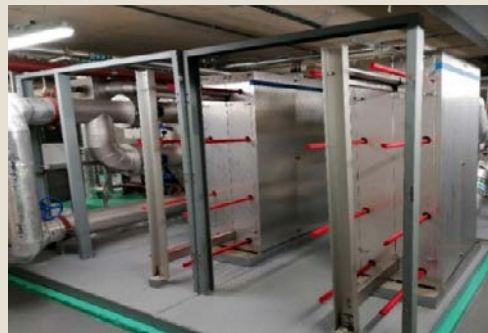
Here East plant room
